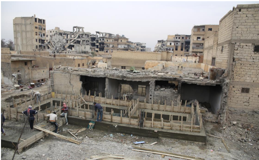
Workmen are rebuilding the Fayad family home, which was destroyed in a Coalition air strike on 12 October 2017 in Raqqa. © Amnesty International
